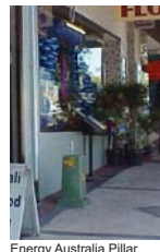
Energy Australia Pillar
