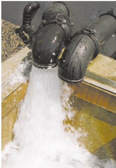
Top right: Water used for weekly fire sprinkler system tests is recycled back into the firewater storage tank for reuse.
