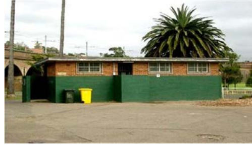
Condition 5 – Very Poor
