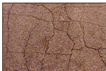
Condition 5 – Very poor
