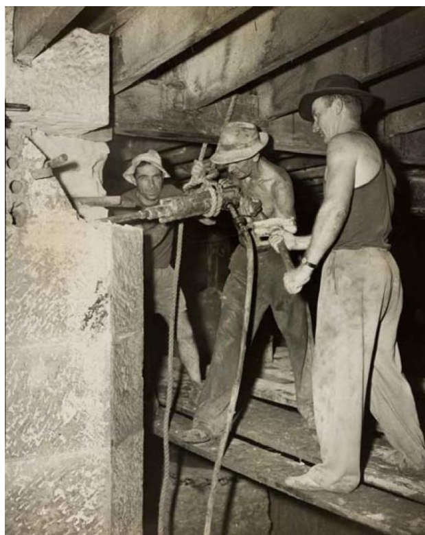
Figure 86 – Building Workmen cutting away the stone piers in the basement for the new centre, 1955.
