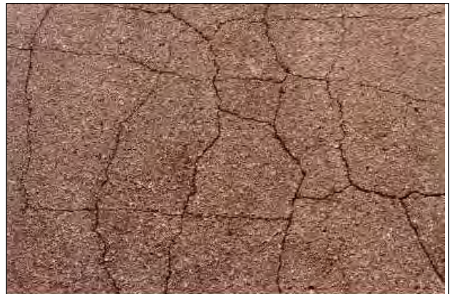
Condition 5 – Very Poor
