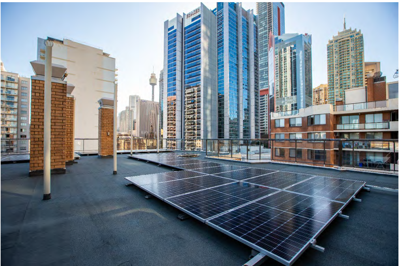
Image 7. Solar panels on the rooftop of the Windsor Plaza apartment building in Sydney city centre. Photo by Katherine Griffiths / City of Sydney
