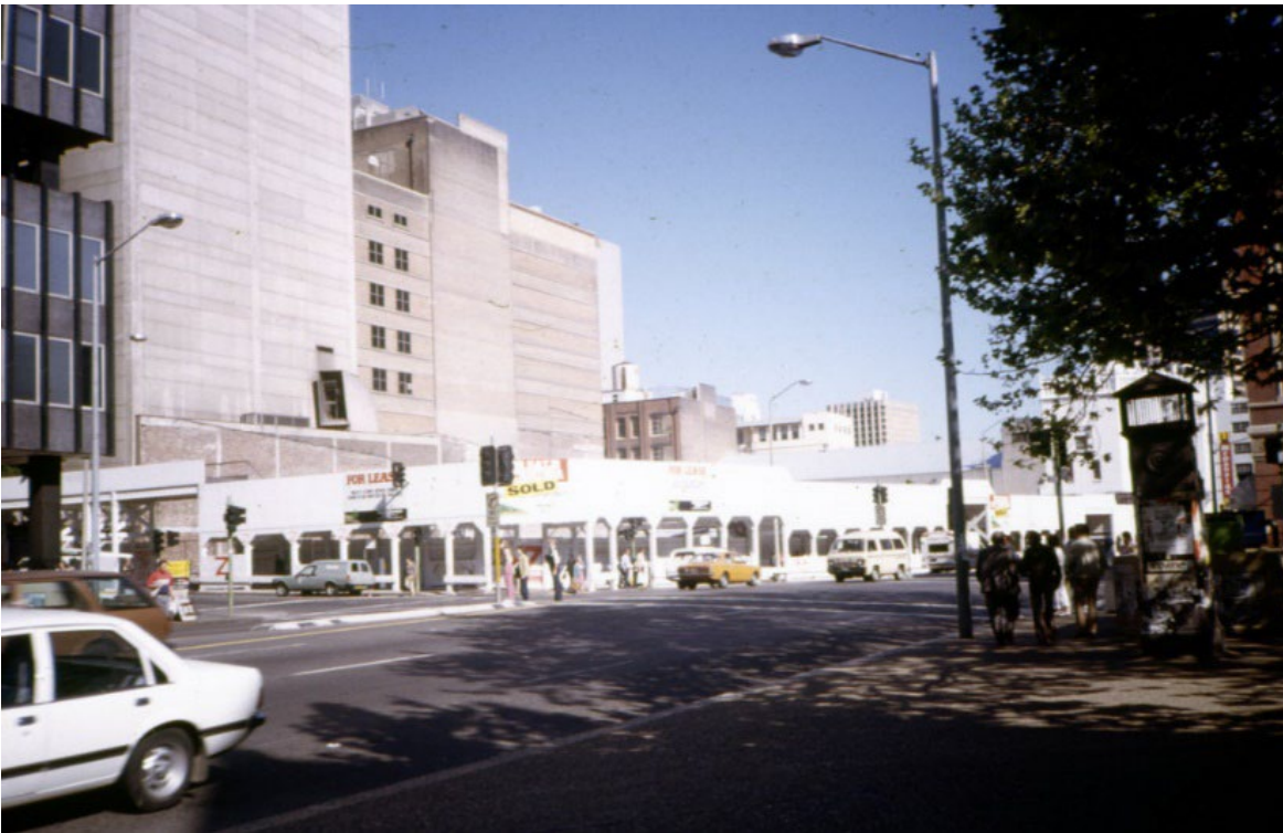
Figure 17 View south east of Tower building site, 580 George Street, Sydney (now HSBC Centre), corner of Bathurst Street, diagonally opposite St Andrew's Cathedral.
