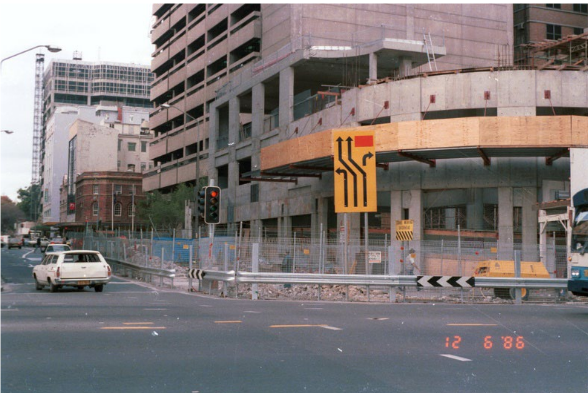
Figure 18 Looking east along Bathurst Street from the corner of George Street and showing the construction of the podium at 580 George Street. Temporary traffic signs are in place.
