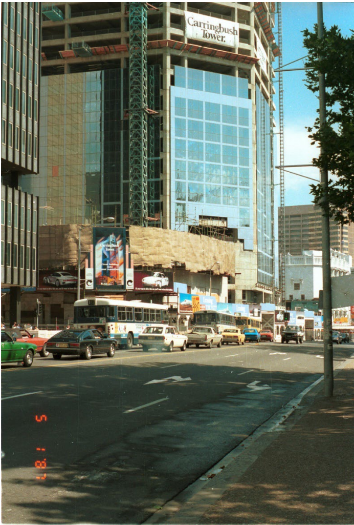
Figure 19 1987 Photograph looking south east from Sydney Square along George Street towards Bathurst Street showing the subject Tower construction site.
