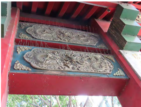
Figure 4.10 Deteriorated plywood of panels D and E on the eastern bay .
