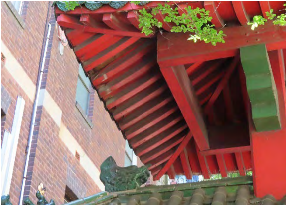
Figure 4.16 Evidence of plywood delaminating from the underside of the curved upper roof of the eastern bay.
