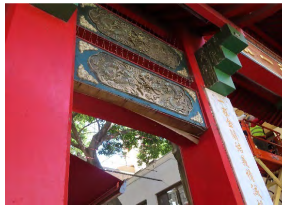
Figure 4.33 Peeling plyboard beneath decorative panel D.
