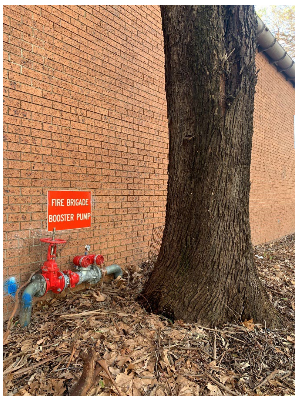
Figure 22 - Tree 25 proximity to existing building
