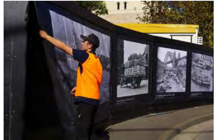
Installing printed vinyl on a 'Type-A' hoarding. Black powder-coated sail track must be used. Photo by City of Sydney.
