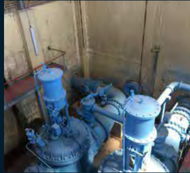
Sydney Water infrastructure
